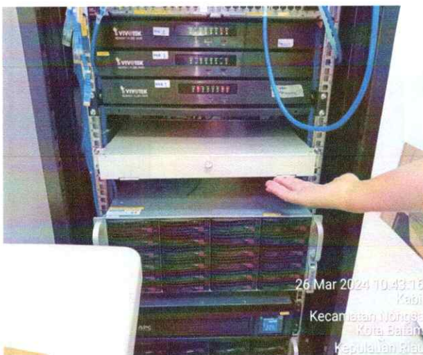
Data center LOT 213
