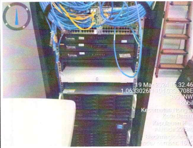
OTB RACK LOT 213
